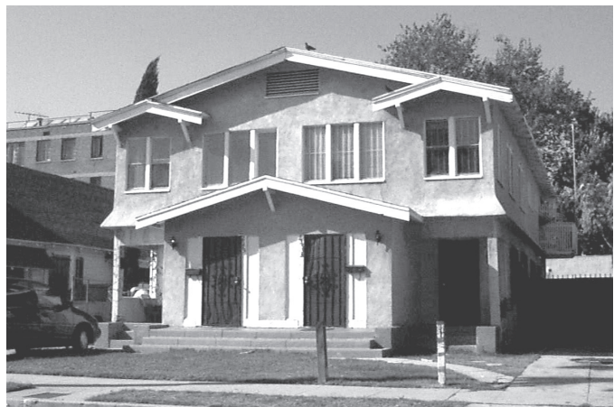
Inappropriate Stucco has been added to this historic structure, covering the wood cladding
