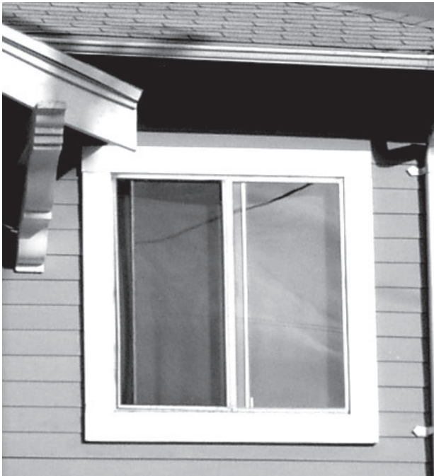
Inappropriate Window Replacement
