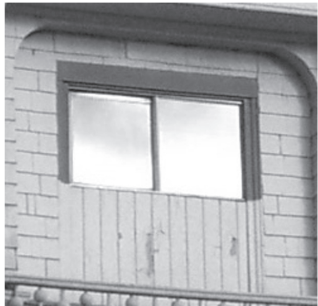
Inappropriate Window Infill
