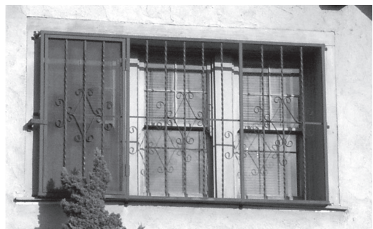
Inappropriate Security Bars
