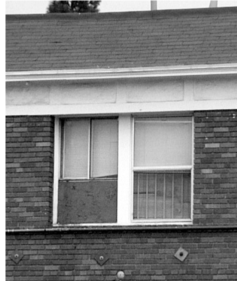
Inappropriate partial window infill
