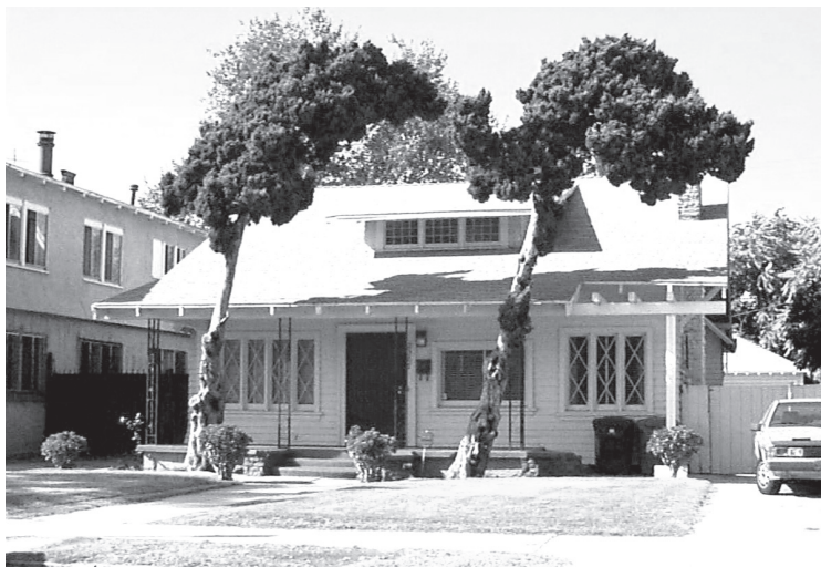
Inappropriate Column Alterations
