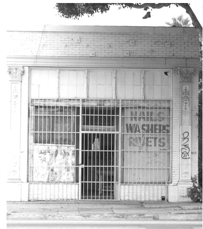
Inappropriate security bars
