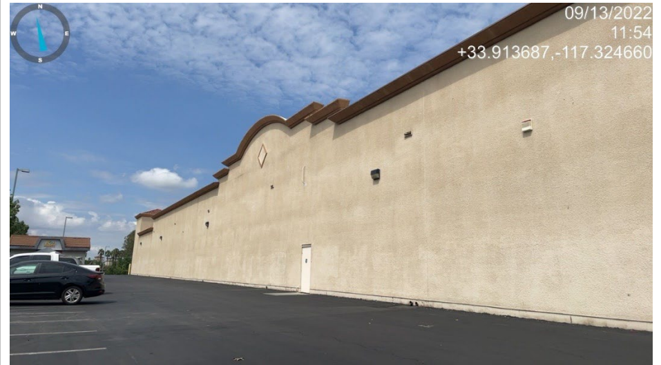
Photo 6: View Northwest of southern side of project site existing structure and active recycling center structure.
